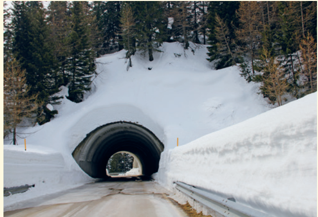
Snow can slide onto the road from steep surfaces over tunnel entrances, as shown here at Lukmanier Pass.
